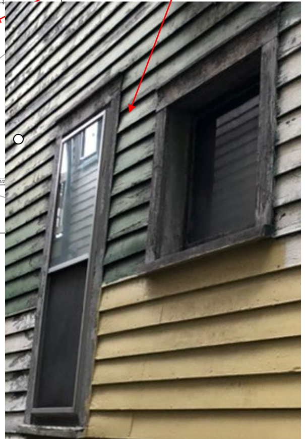
Applicant photo. East elevation. This close-up view shows the window casings for typical vertical window openings; the protruding trim at the headers and sills is also visible.
