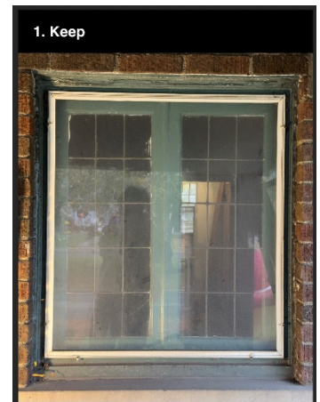
Site Photo 5, by Applicant, October 2023: (North) front elevation, first floor next to front door, showing original wood casement behind storm window to remain.
