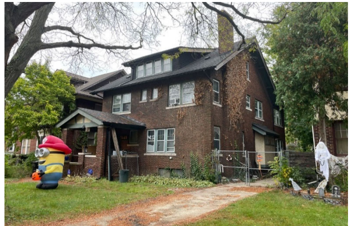
Site Photo 3, by Staff, October 19, 2023: (East) side elevation of house, showing original wood windows behind storm windows.
