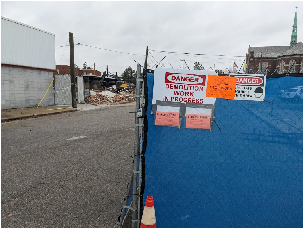
View of site conditions during demolition activity, including City of Grosse Pointe Park building permits (in pink) and City of Detroit Stop Work order (in orange). The extant Jefferson-fronting DPW building, partially demolished later that spring, is visible at left. Staff photo, March 31, 2023.
