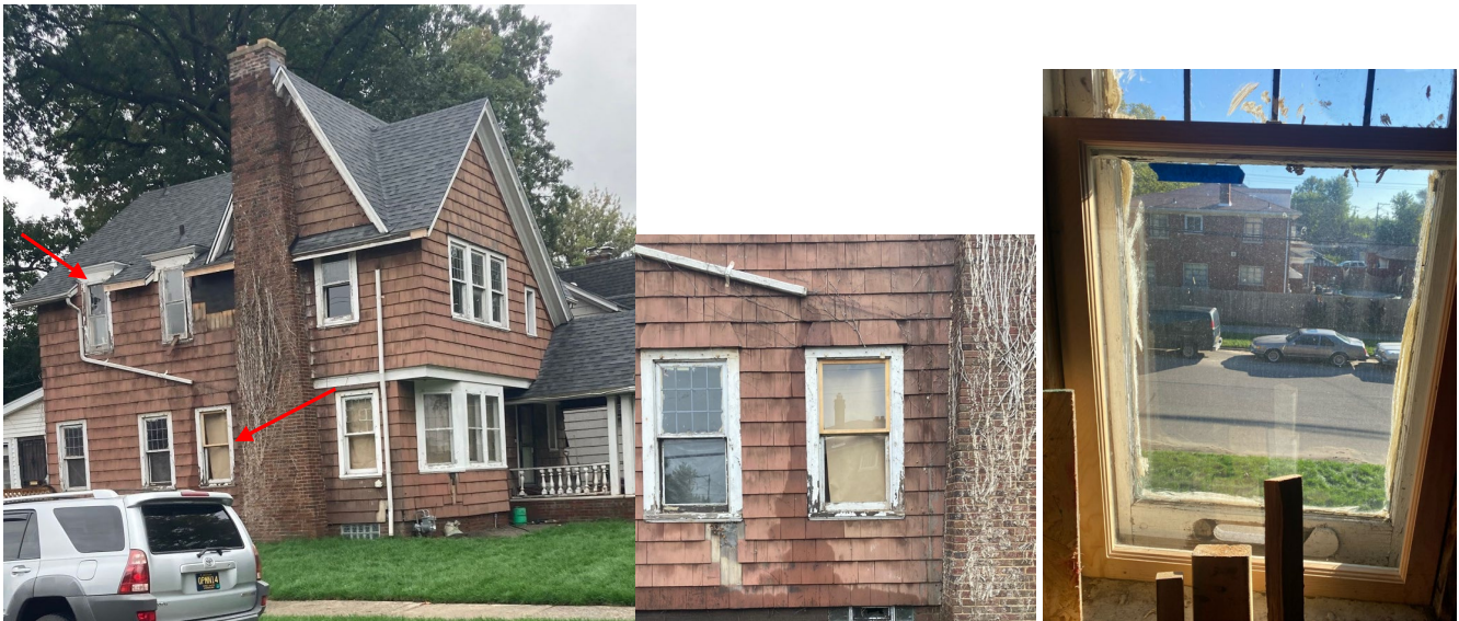
East Wall: One upper sash of a window on the lower story, and one lower sash at the second story have been replaced with new custom wood sash. The prior condition of the window is not visible due to extensive vegetation.
