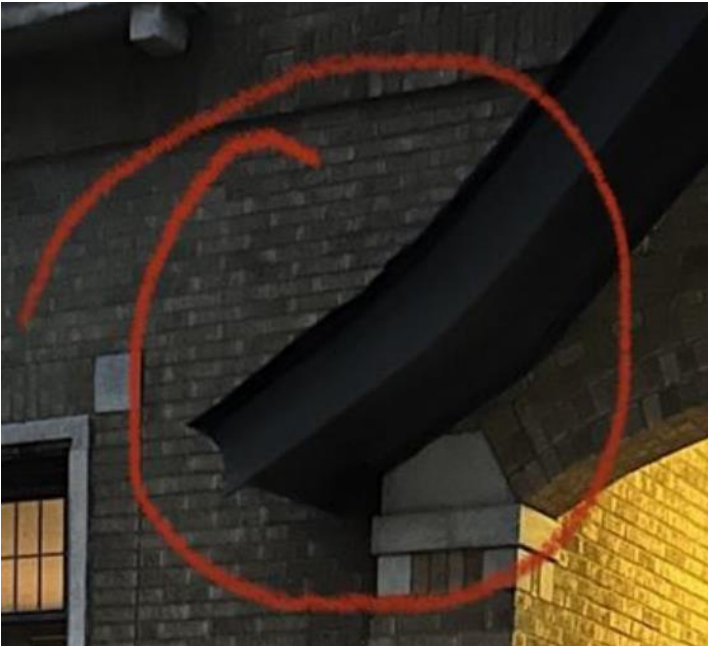
Detail of current condition (typical of all four locations). Photo provided by applicant, cropped by staff to highlight pertinent area.
