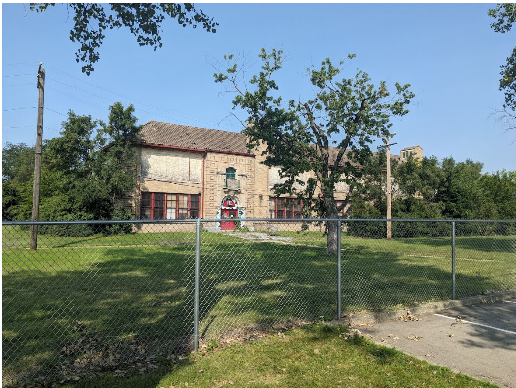
View of east elevation (on vacated Wisconsin Street), nominally described as the "front" elevation in the HDAB Report. Diseased tree is in approximate location of new building footprint. Staff photo, September 1, 2023.
