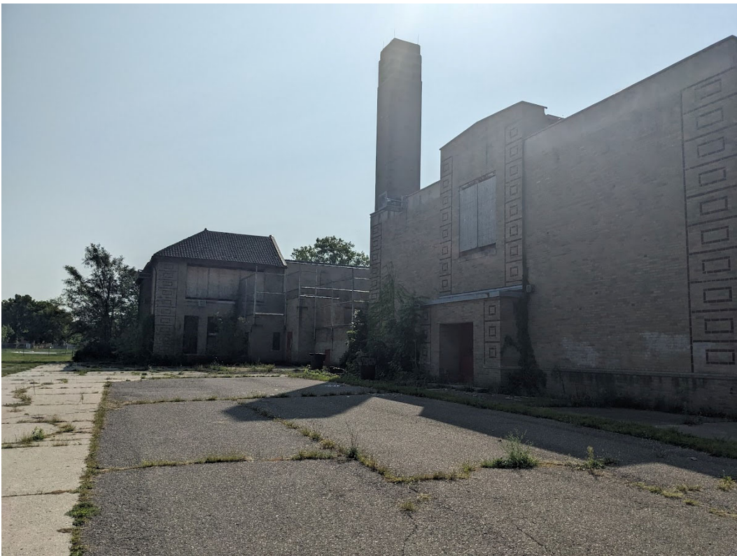
Existing conditions at the rear, showing areas of flat roof and utility parking lots. Staff photo, September 1, 2023.
