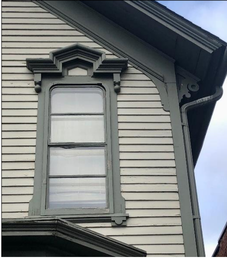
The front window openings are deeply detailed with elaborate window hoods, two-over-two double-hung windows with upper sash rounded corners, and dimensional/profiled window casings and sill brackets.
