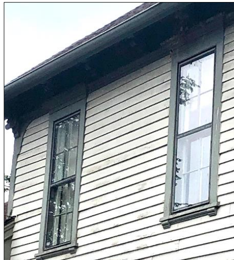
The side window openings have narrow rectangular projecting hoods, four-over-four double-hung windows with rectangular corners, flat and straight-edged window casings, and simplified, yet still dimensional, sill brackets.
