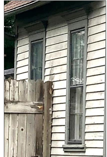
The window openings on the extension have window hoods and double-hung windows similar to the main house's side windows, but the sills have utilitarian trim pieces instead of decorative brackets.
