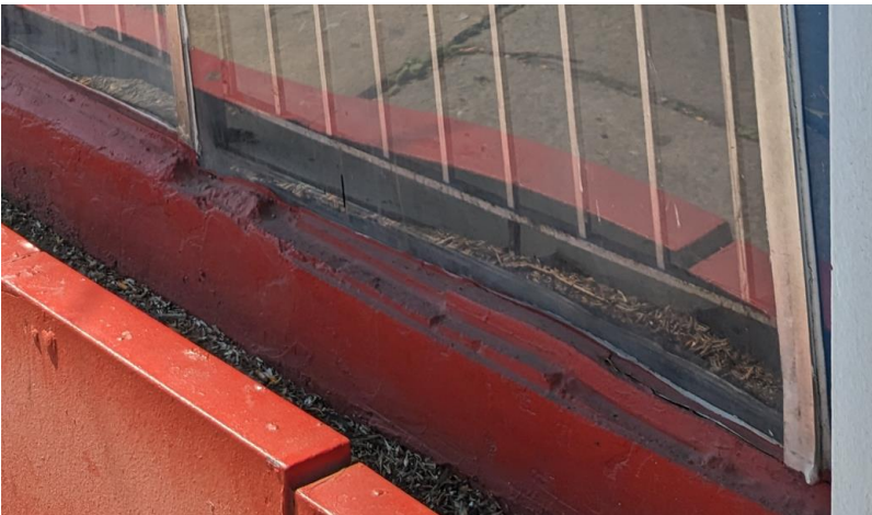
Example of window damage. August 2023 photo by staff.
