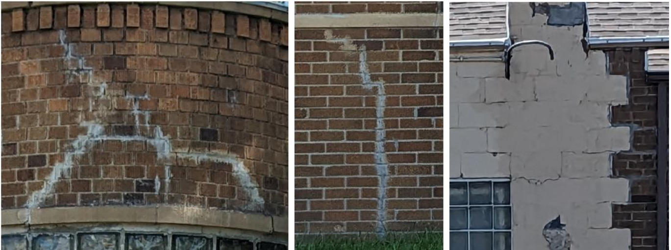
Representative areas of damage and prior repair. August 2023 photos by staff.
