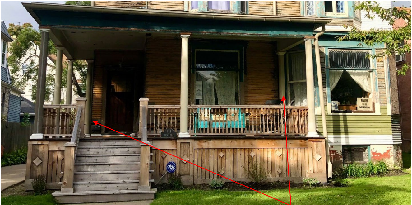
HDC staff photo, August 30, 2023. Full columns were installed in place of reinstalling historic pilasters. Photos of pilasters in their original locations are on the following page.
