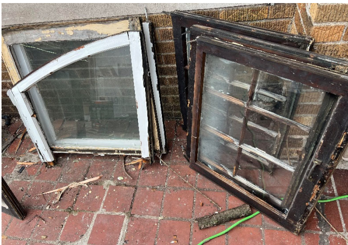
Site Photo 5, by Applicant, showing conditions of original windows removed. The archtop window shown here may be from the window pair discussed on the next page.
