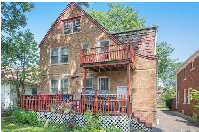
Site Photo 3, by Applicant (unknown date) March 22, 2023: (South) rear elevation, showing original windows.
