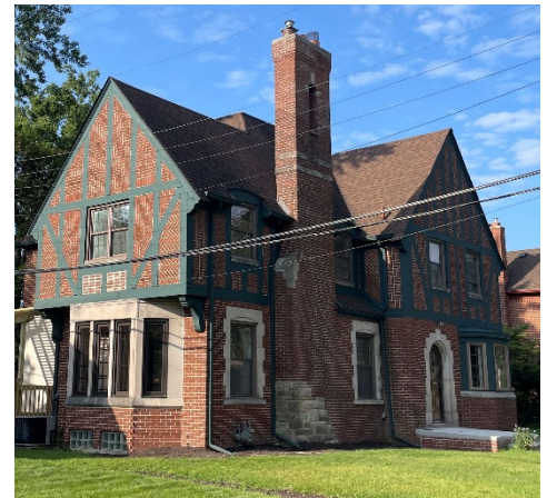
Site Photo 9, by Staff, August 29, 2023: East (side) and north (front) elevation showing tuckpointing below second floor window and front porch (completed without approval).
