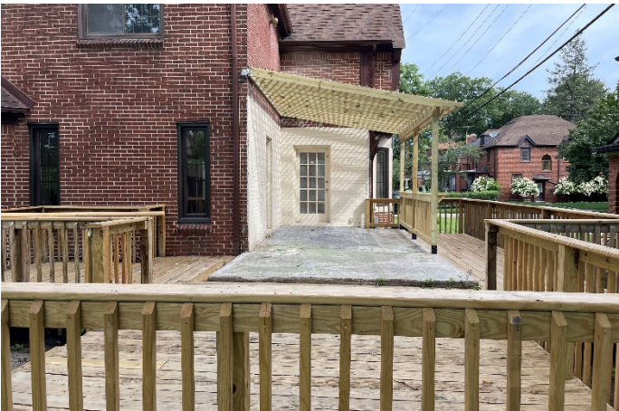
Site Photo 2, by Staff, August 14, 2023: South elevation of former room expansion by previous owner without approval and construction of the new pergola by current owner without approval. The surrounding deck and railing were repaired by current owner.
