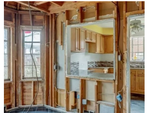
Site Photo 6, by realtor.com, April 2023: Dining room bay and kitchen interior showing steel casement windows that were replaced by the current owner.
