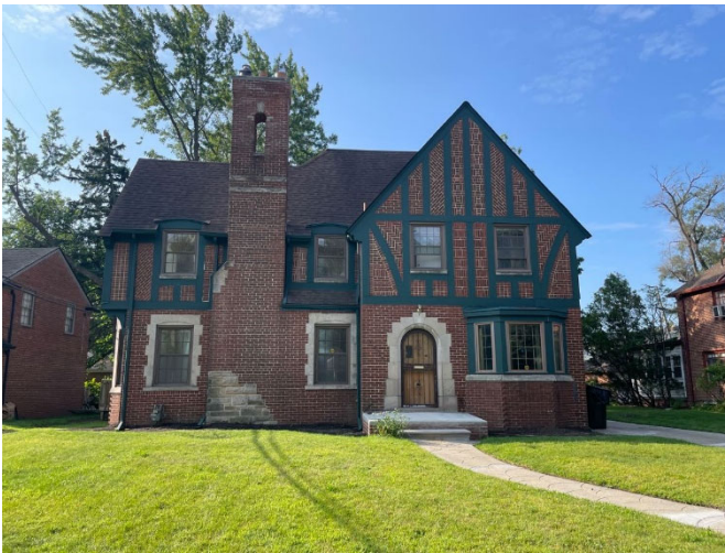
Site Photo 1, by Staff August 29, 2023: (North) front elevation of house, showing location of removed foundation plantings and painted trim, work completed without approval.
