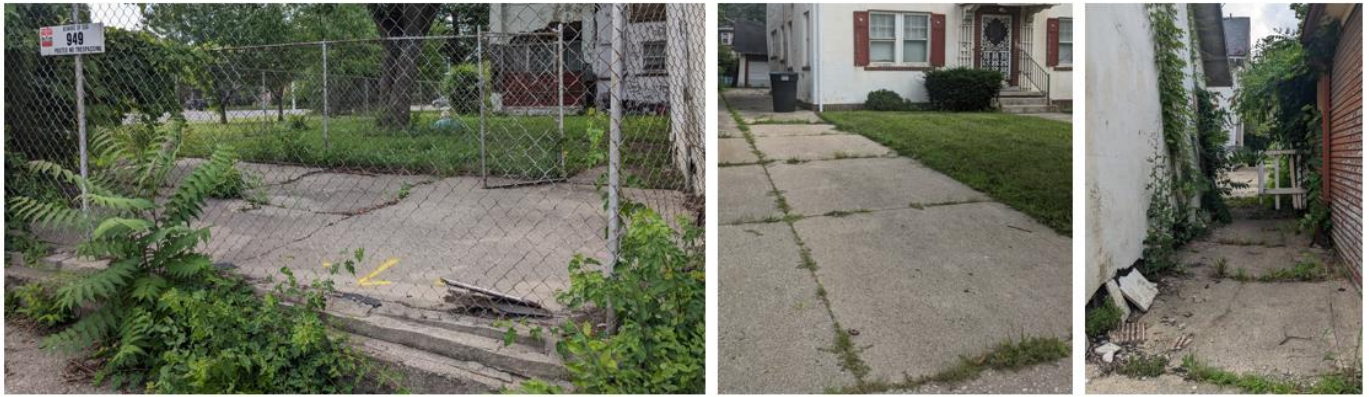
Areas of concrete proposed for replacement. August 2023 photos by staff.
