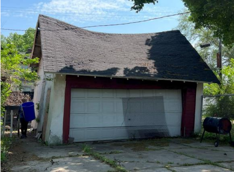
Photo by applicant indicating non-historic steel door and structural damage.
