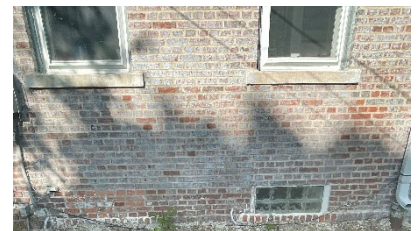
Site Photo 7, by Staff, August 2, 2023: (west) side elevation, showing paint removal work.
