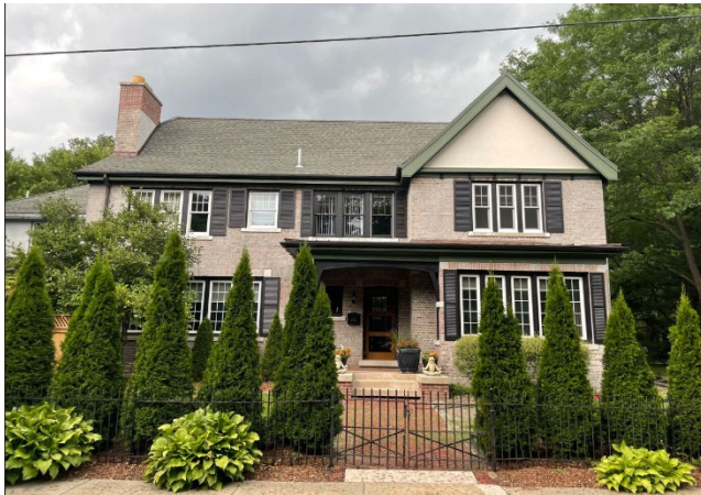
Site Photo 1, by Staff July 20, 2023: (Southeast) front elevation, showing vinyl windows from a previous owner and some wood windows.
