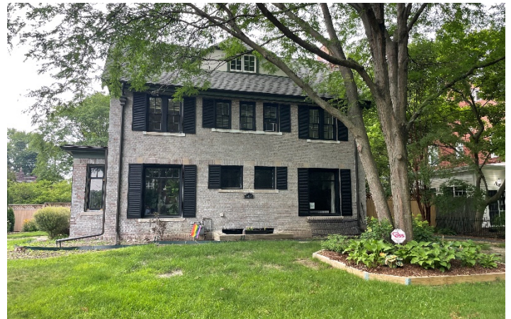
Site Photo 2, by Staff July 20, 2023: (Northeast) side elevation, showing two fixed picture windows that replaced vinyl windows. These windows received a Denial from the previous application in June 2023. Vinyl windows on the 3 rd floor were installed by a former owner.
