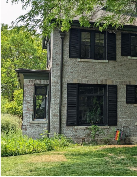
Site Photo 5, by Staff June 5, 2023: (Northeast) side elevation, detail of window #7 a newly constructed 2/1 wood window.
