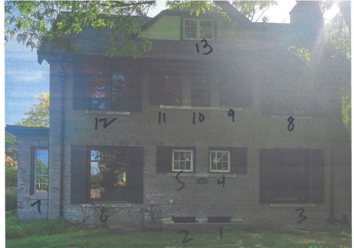
Figure 1, by Applicant: (Northeast) side elevation, picture windows #3 and #6, and replaced vinyl window #7.
