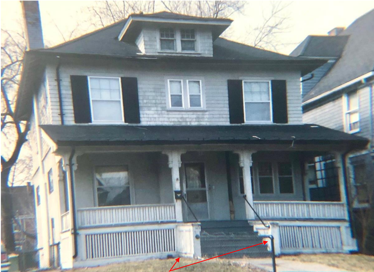
1983 Designation photo, HDAB. Wing walls that were removed without Commission approval.
