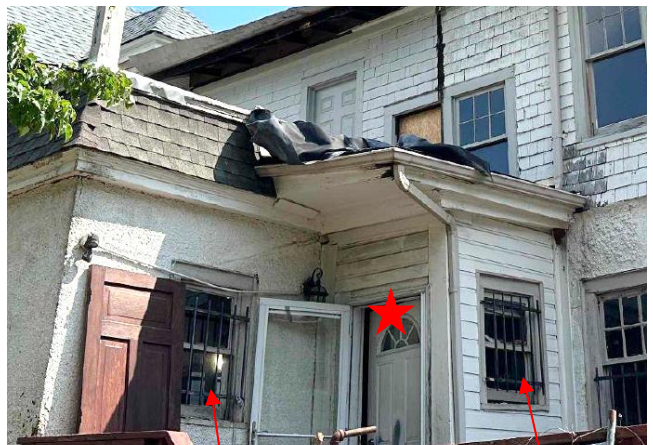
Window to be removed; French door to be installed. New window location. Window to remain.
