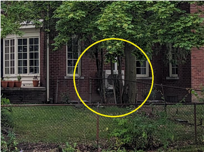
Ground-level unit on east wall viewed from Rosa Parks sidewalk towards back yard of house.
