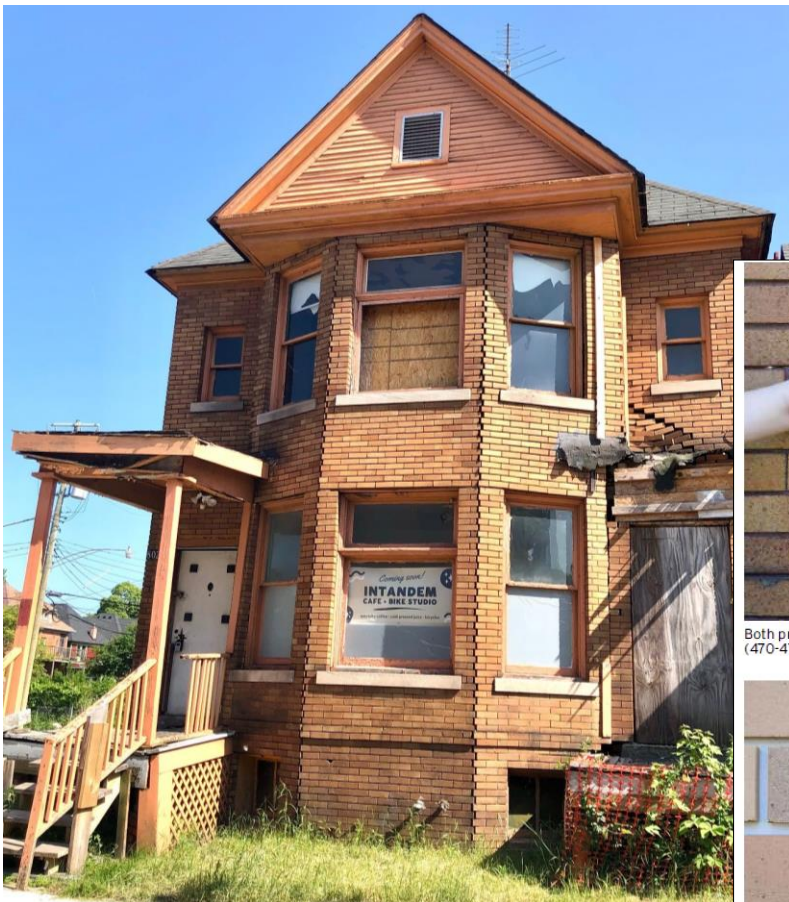
Staff photo, May 30, 2023. Applicant photo of brick samples.
