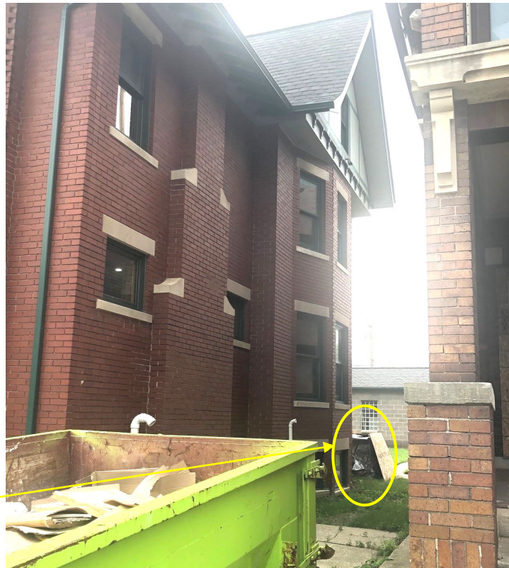
Right: Staff photo, June 29, 2023. Condensing units are circled in yellow.
