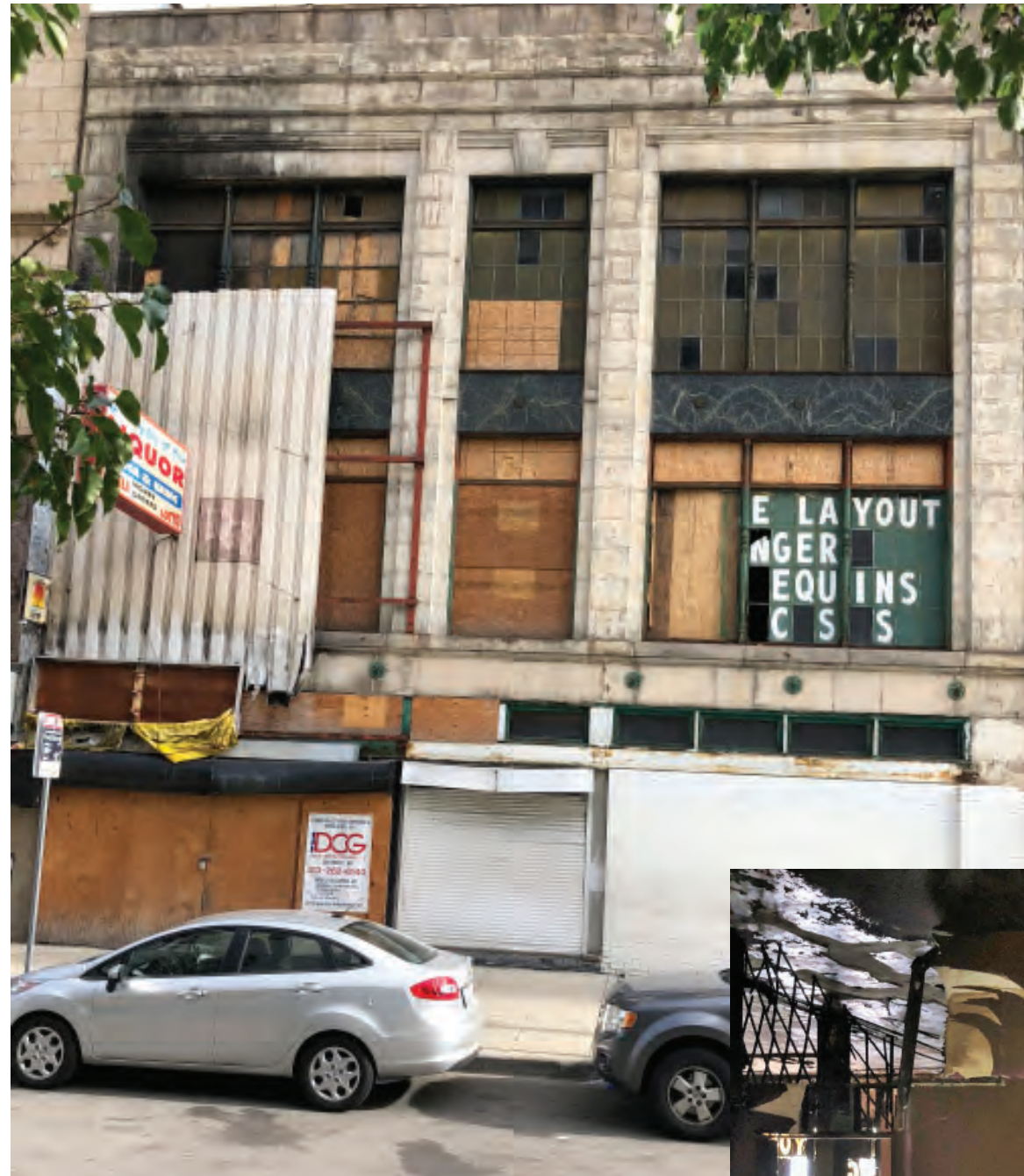
1332-1336 BROADWAY FIRE DAMAGE ON BOTH 2ND & 3RD FLOORS
