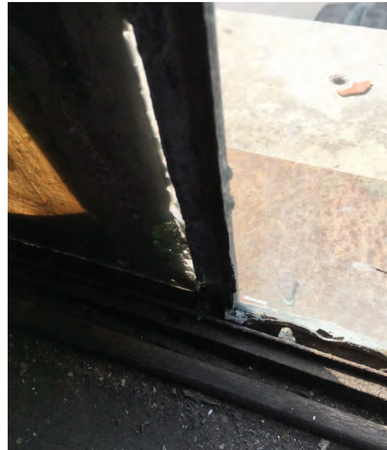
1332-1336 BROADWAY DAMAGED CAMING
