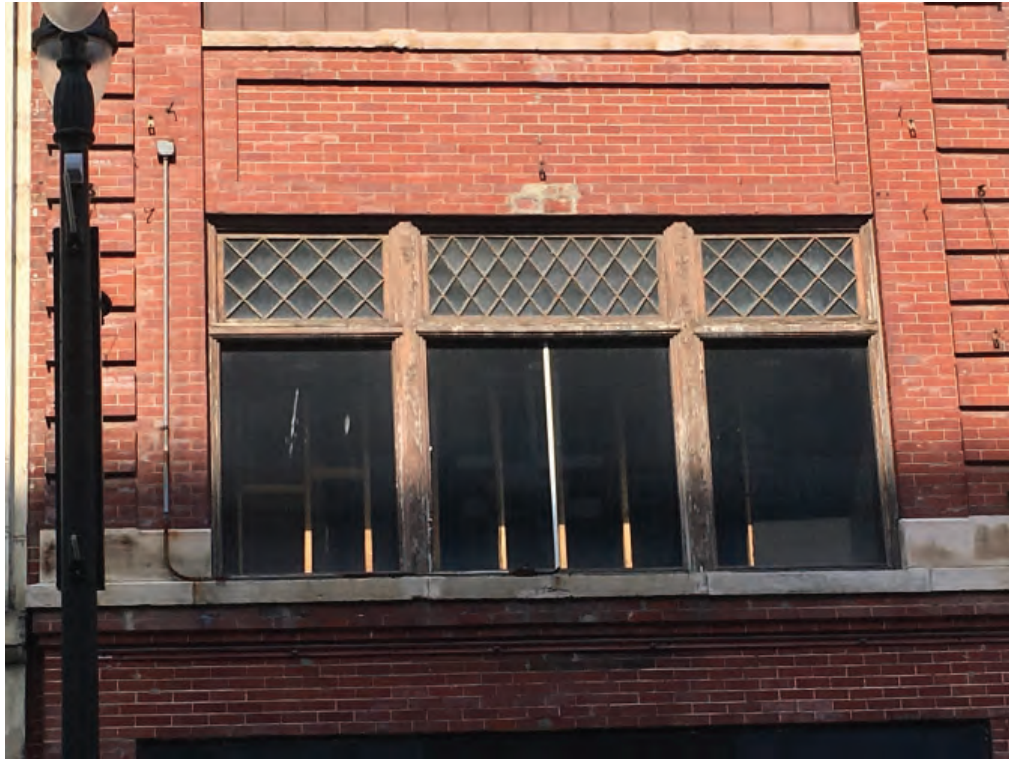
1326 BROADWAY 2ND STORY WOOD WINDOWS. LOWER SASH HAS BEEN REMOVED AND REPLACED WITH FIXED GLASS.
