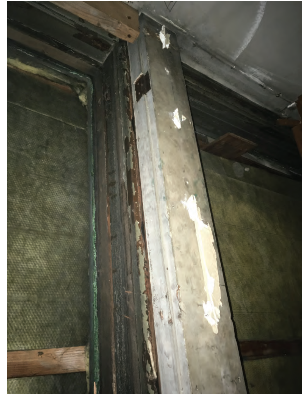
1326 BROADWAY 3RD STORY WINDOW OPENING FROM INTERIOR WITH PLYWOOD REMOVED. WINDOW FRAMES REMAIN; SASH IS MISSING.
