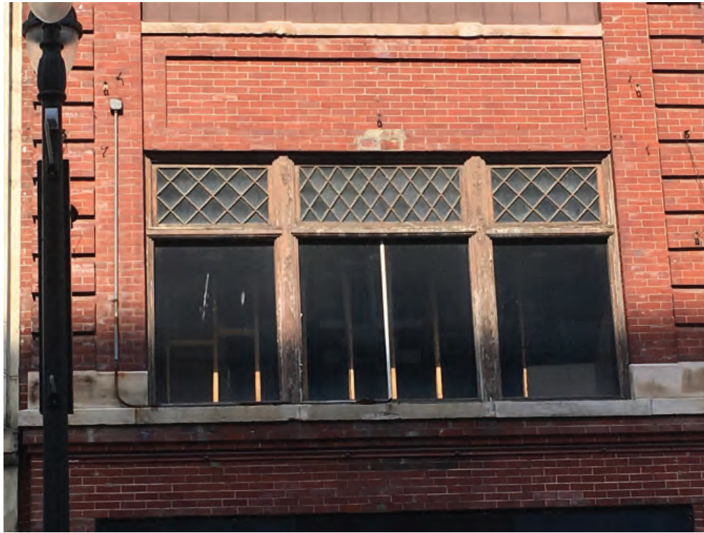
1326 BROADWAY 2ND STORY WOOD WINDOWS. LOWER SASH HAS BEEN REMOVED AND REPLACED WITH FIXED GLASS.
