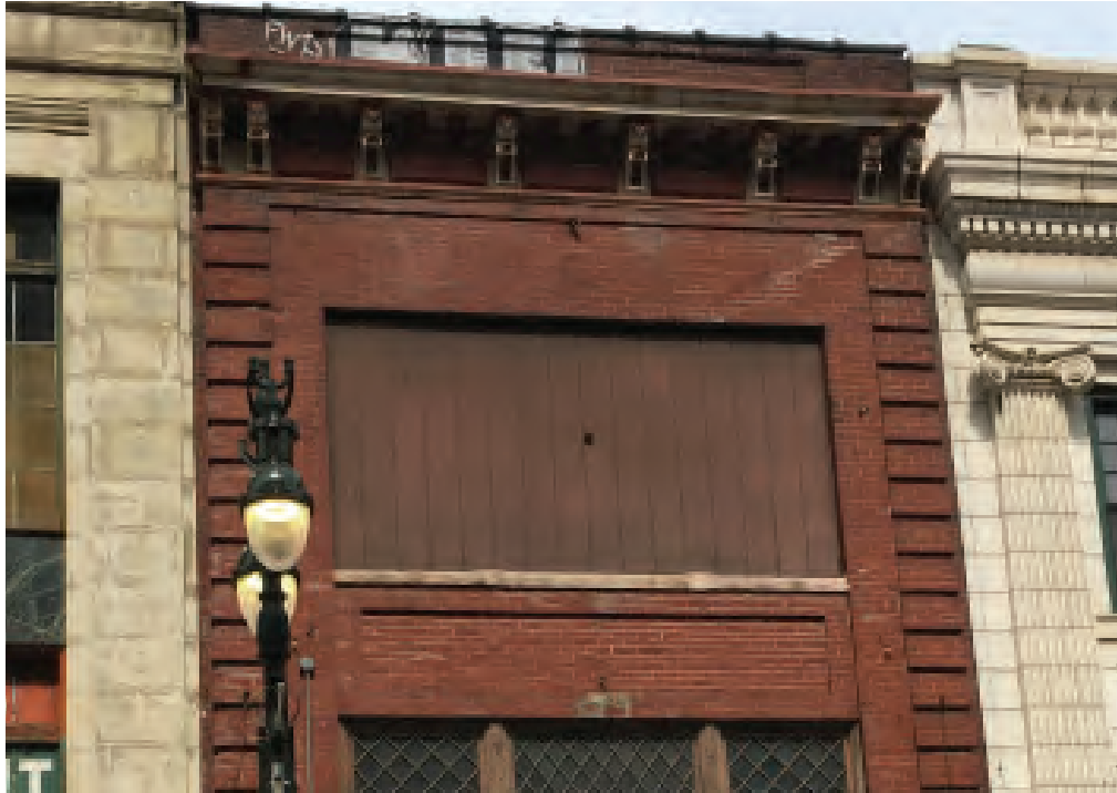
1326 BROADWAY 3RD STORY WINDOW OPENING HAS BEEN BOARDED OVER.
