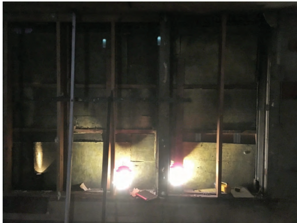
1326 BROADWAY 3RD STORY WINDOW OPENING FROM INTERIOR WITH PLYWOOD REMOVED. WINDOW FRAMES REMAIN; SASH IS MISSING.
