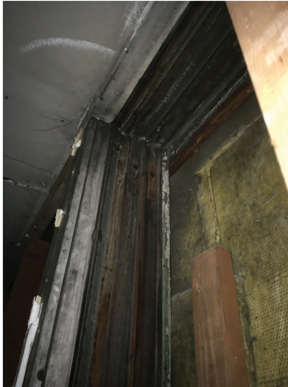
1326 BROADWAY 3RD STORY WINDOW OPENING FROM INTERIOR WITH PLYWOOD REMOVED. WINDOW FRAMES REMAIN; SASH IS MISSING.
