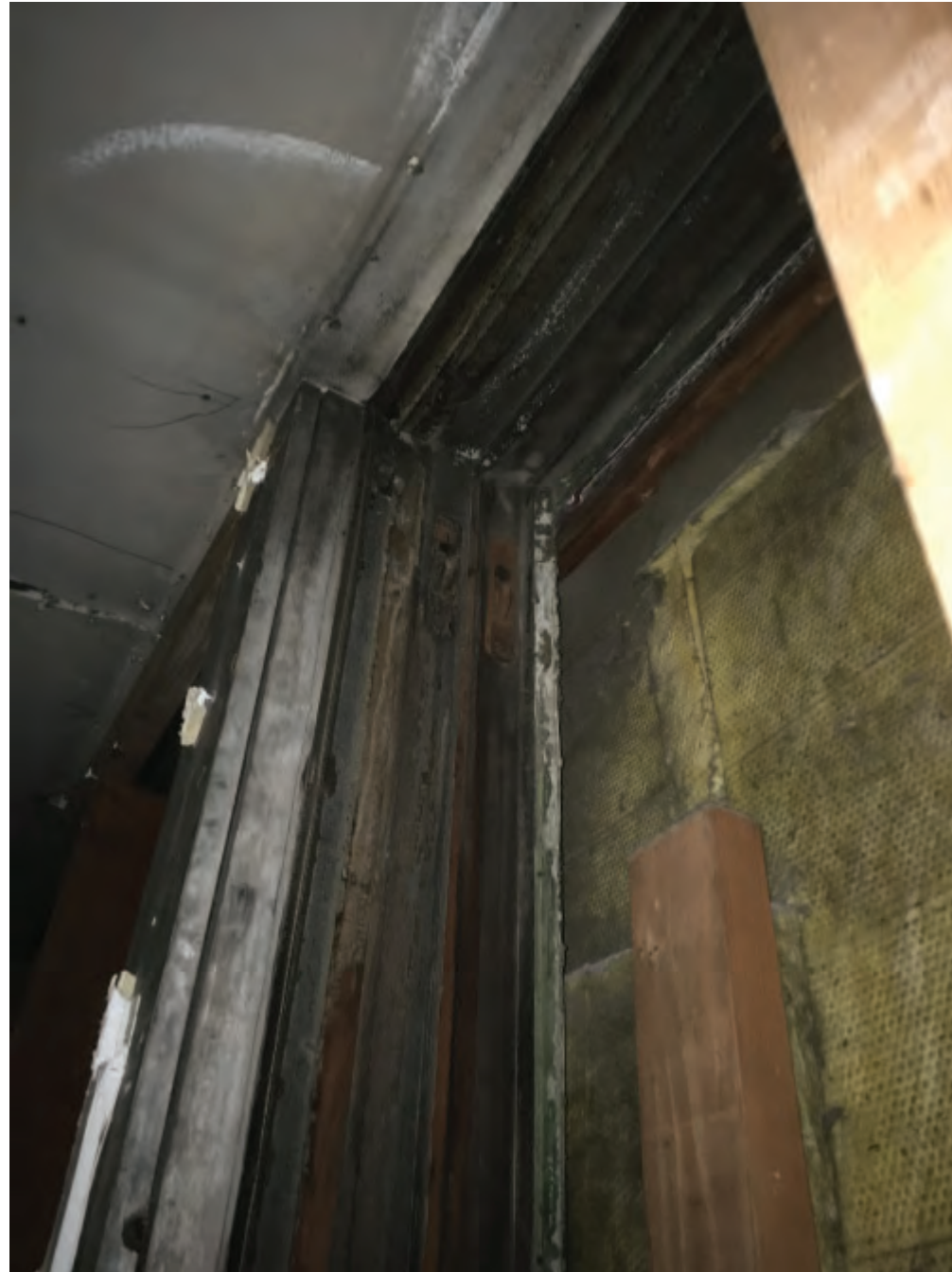
1326 BROADWAY 3RD STORY WINDOW OPENING FROM INTERIOR WITH PLYWOOD REMOVED. WINDOW FRAMES REMAIN; SASH IS MISSING.
