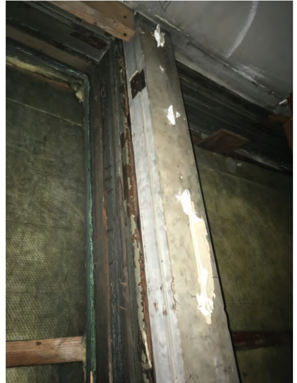
1326 BROADWAY 3RD STORY WINDOW OPENING FROM INTERIOR WITH PLYWOOD REMOVED. WINDOW FRAMES REMAIN; SASH IS MISSING.
