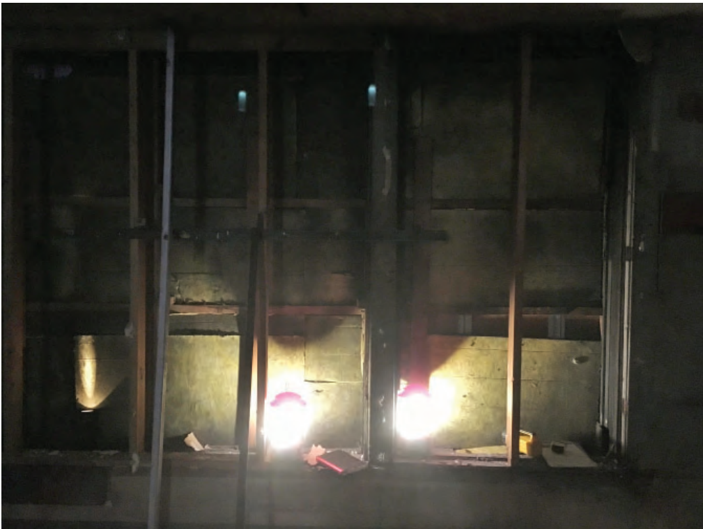
1326 BROADWAY 3RD STORY WINDOW OPENING FROM INTERIOR WITH PLYWOOD REMOVED. WINDOW FRAMES REMAIN; SASH IS MISSING.
