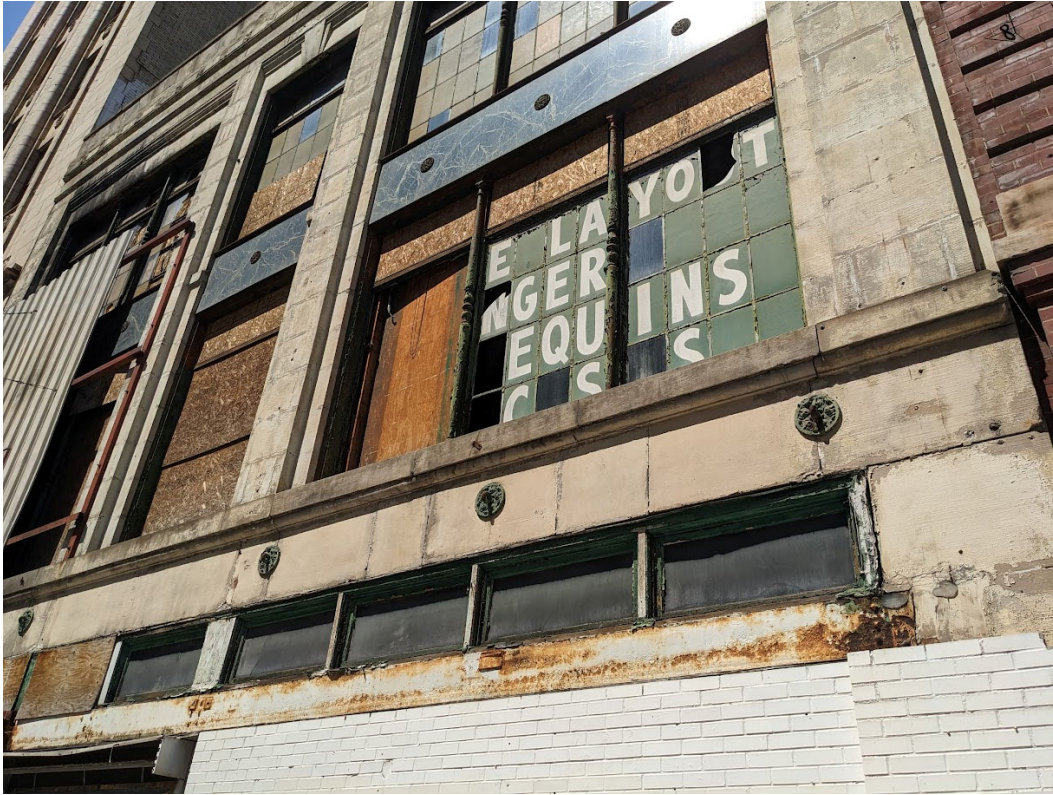
Detail view of the façade at 1332-1336 Broadway. Visible are the incorrectly treated mortar joints, evidence of water infiltration, and several historic elements (cast iron posts, medallions, stone panels) intended to be salvaged and reused. Staff photo, May 31, 2023.
