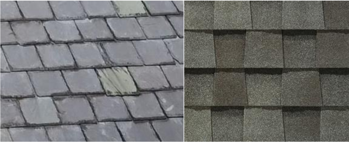
Left: Existing roof. Right: Proposed replacement product. Image from submitted application materials.
