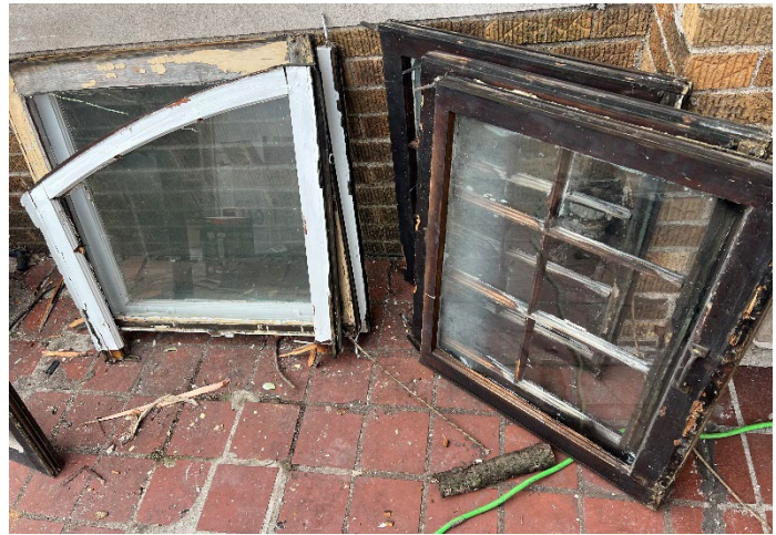
Site Photo 5, by Applicant, showing conditions of original windows removed.
