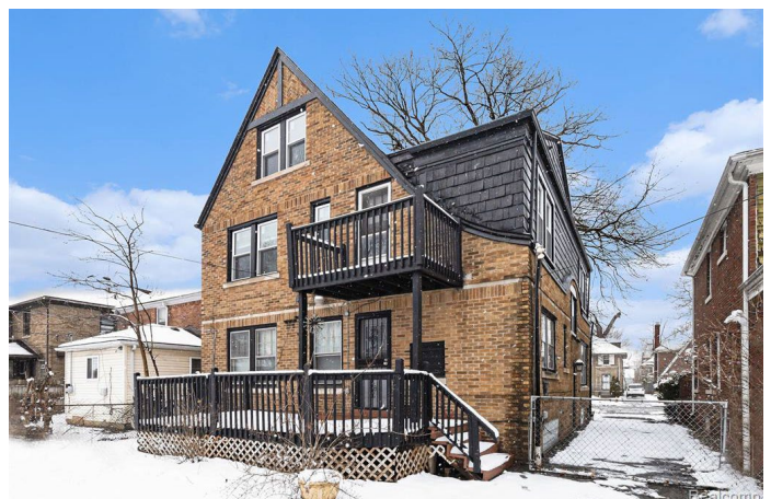
Site Photo 4, by Applicant 2022: (South) rear elevation showing replaced windows, repaired siding, new railings, and trim/siding paint work. Notice windows on 2 nd and 3 rd floor have been replaced, while the original first-floor windows remain.
