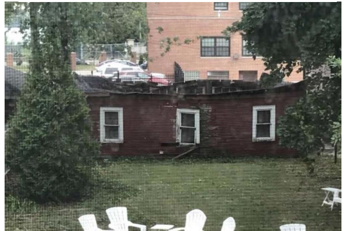
Site Photo 3, by applicant September 2018: (facing south) north elevation of garage, showing roof collapse and wood framing failure.
