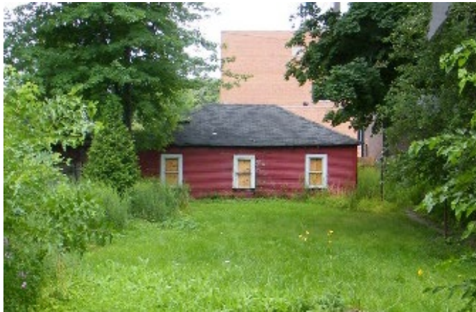
Site Photo 2, by applicant June 2013: (facing south) north elevation of garage, showing previous condition.
