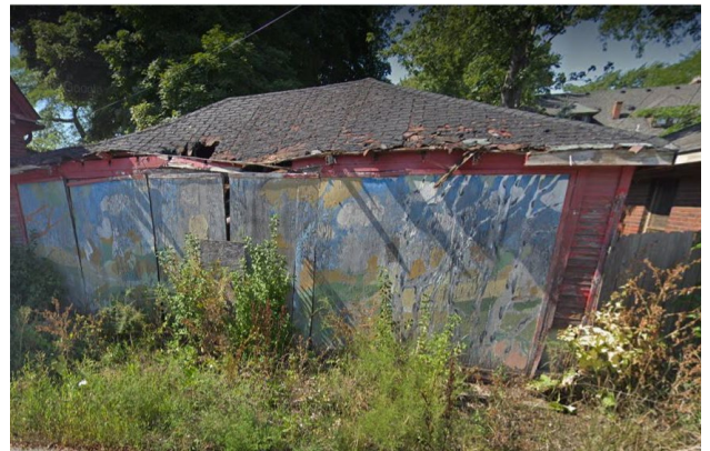
Site Photo7, by Google Streetview August 2018: (Facing north) former garage from rear alley, showing conditions one month prior to roof collapse.
