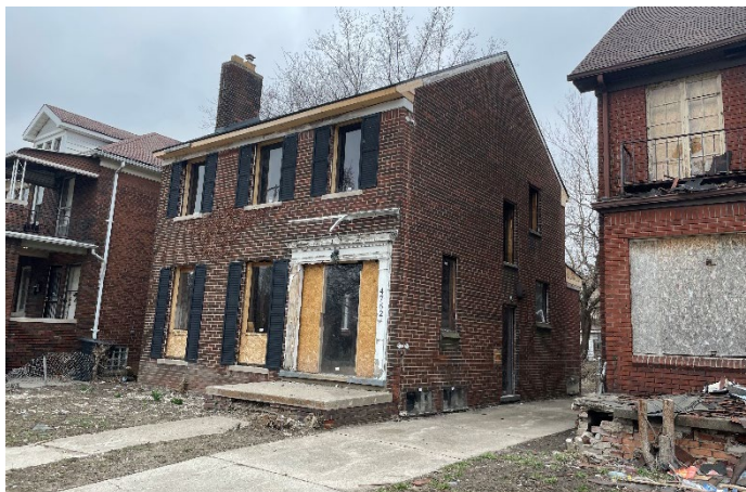
Site Photo 3, by Staff March 22, 2023: (South) front elevation, showing secure view and boarding on windows and side door missing on east elevation.
