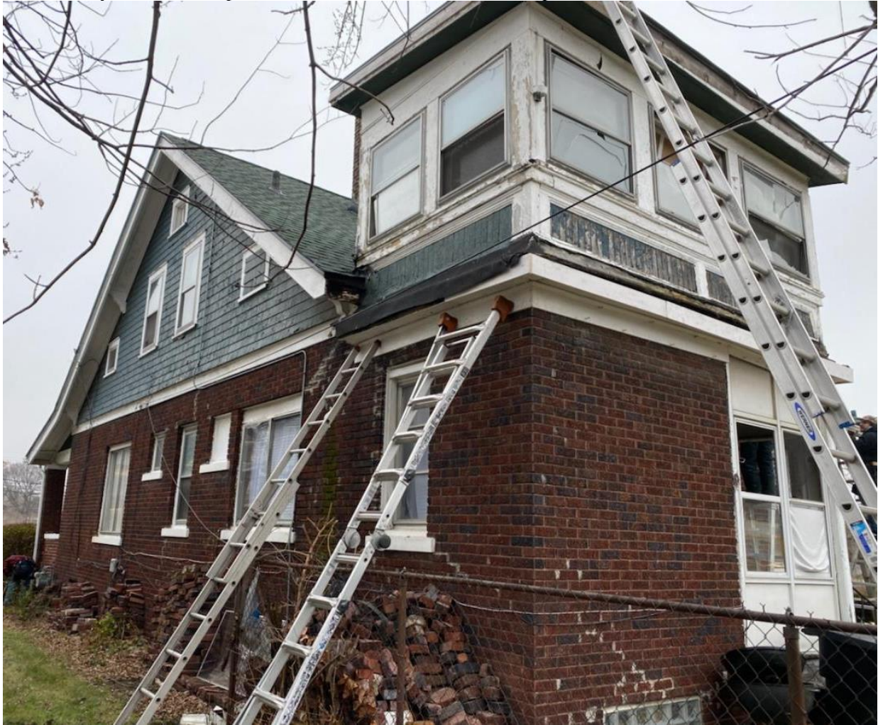
2020 applicant photo provided with gutter replacement application.
