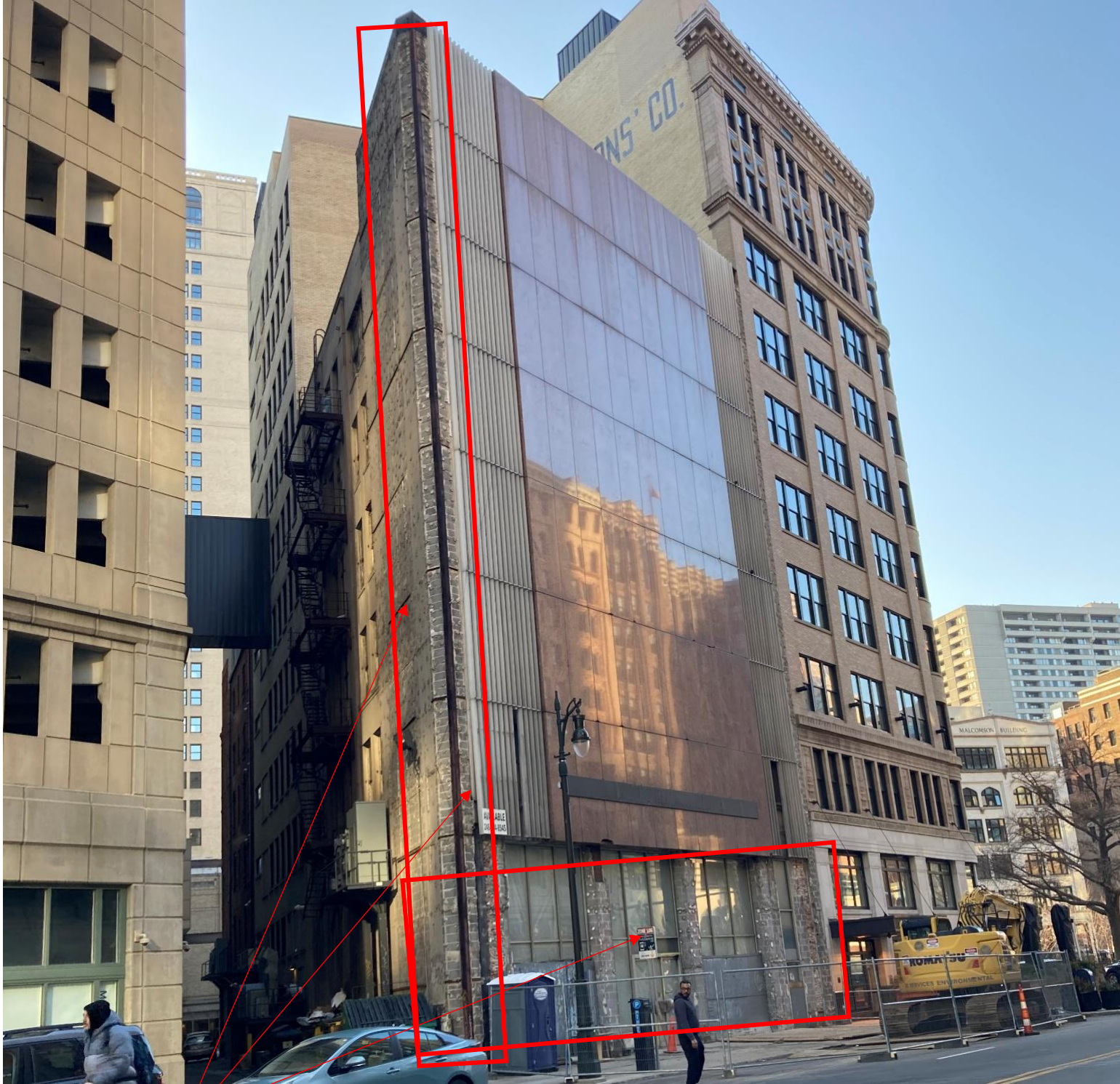
Current appearance. Note that marble has been removed from these locations
