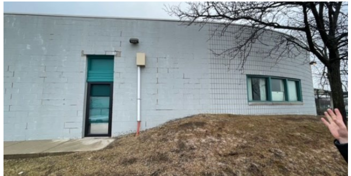
Site Photo 2, by Staff February 23, 2023: (South) Side entrance showing location of wall where louver is proposed to the upper right of the utility box.
