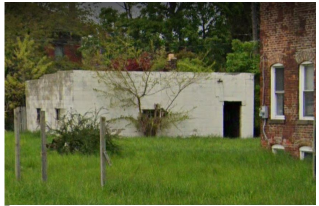
Site Photo 4, by Google Street May,2019: (Northwest) Rear elevation, showing rear garage prior to demolition.
