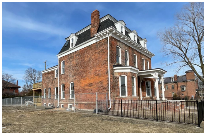
Site Photo 3, by Staff February 20, 2023: (West) side elevation, showing front and rear fence installations, and former site of rear garage (work completed without approval).
