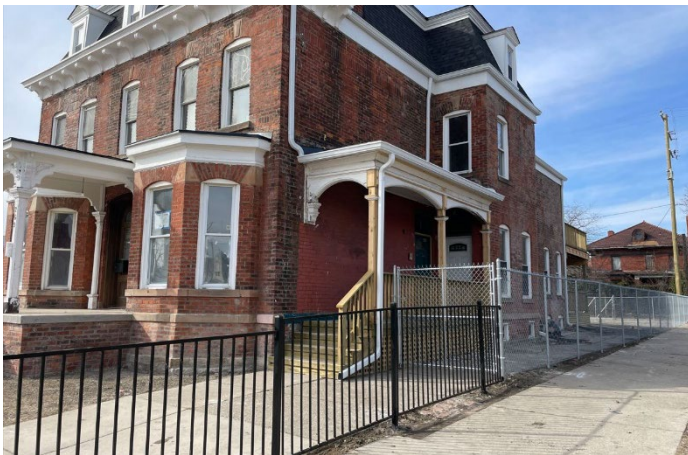
Site Photo 2, by Staff February 20, 2023: (East) side elevation, showing front and rear fence installations, east porch installation (work completed without approval).
