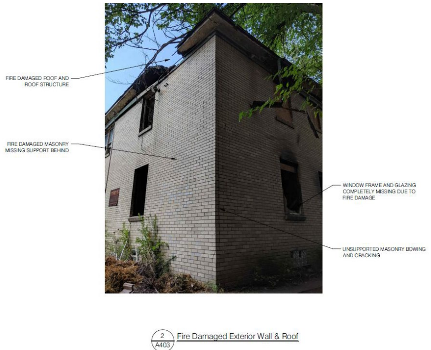
Figure 3, by BSEED e-Plans BLD2019-06541: East Courtyard (East) north elevation, showing fire damaged window openings prior to work on brick wall, window openings, and roof.
