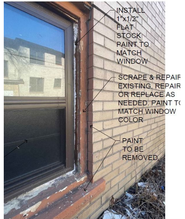
Detail photo 2, by applicant: Showing exposed brick mould after brake metal was removed. Application proposes to repair wood, scrape and repaint wood, and caulk where needed.
