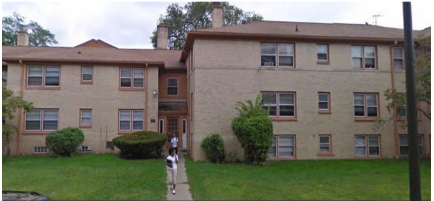
Site photo 4, by Google Street, September 2009: Whitmore (North) elevation, showing 2/2 horizontal muntin, double hung wood windows.
