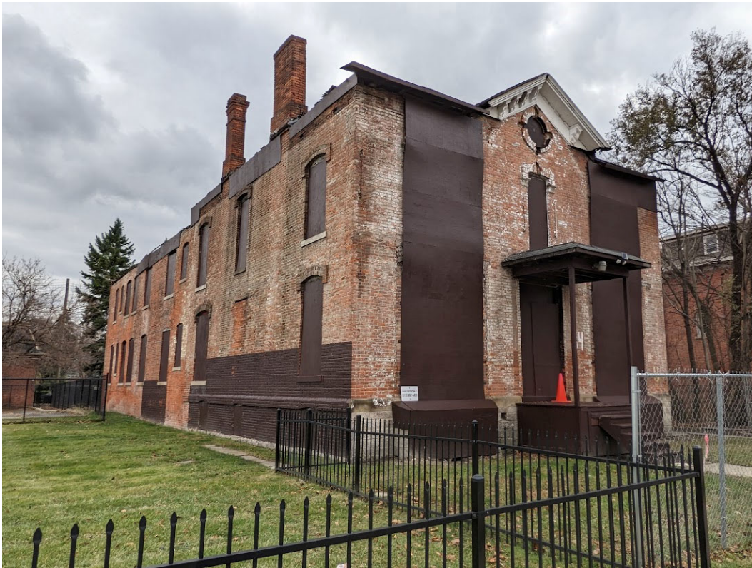
View of vacant 64 Edmund Place, immediately east of the subject parcel. Staff photo, November 28, 2022.
