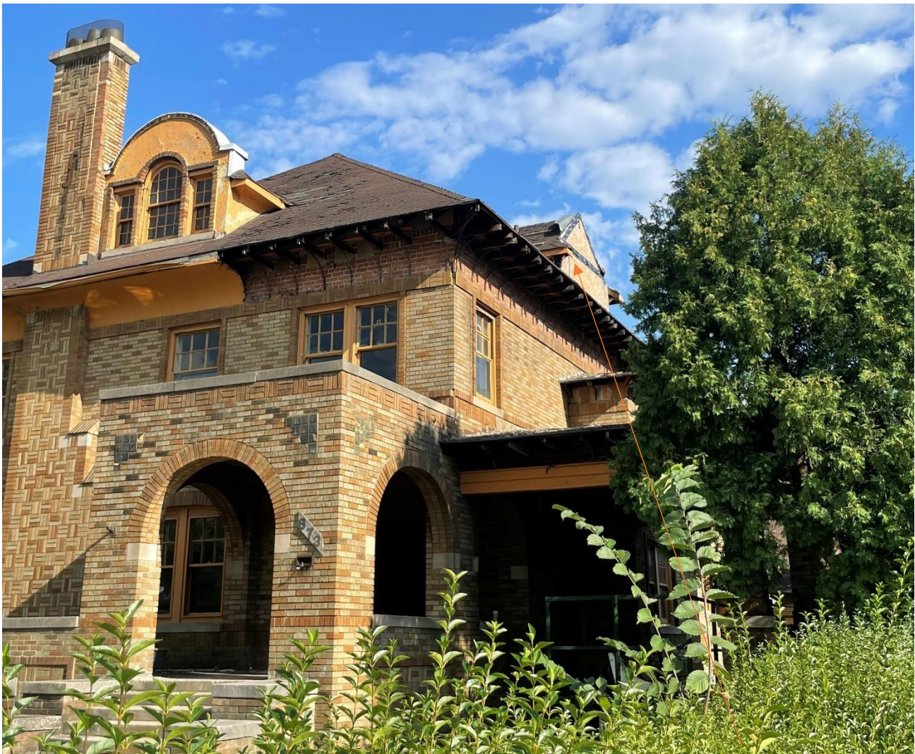
Photo taken by HDC staff in 8/2022 to illustrate unapproved removal of stucco from the side/west elevation dormer
