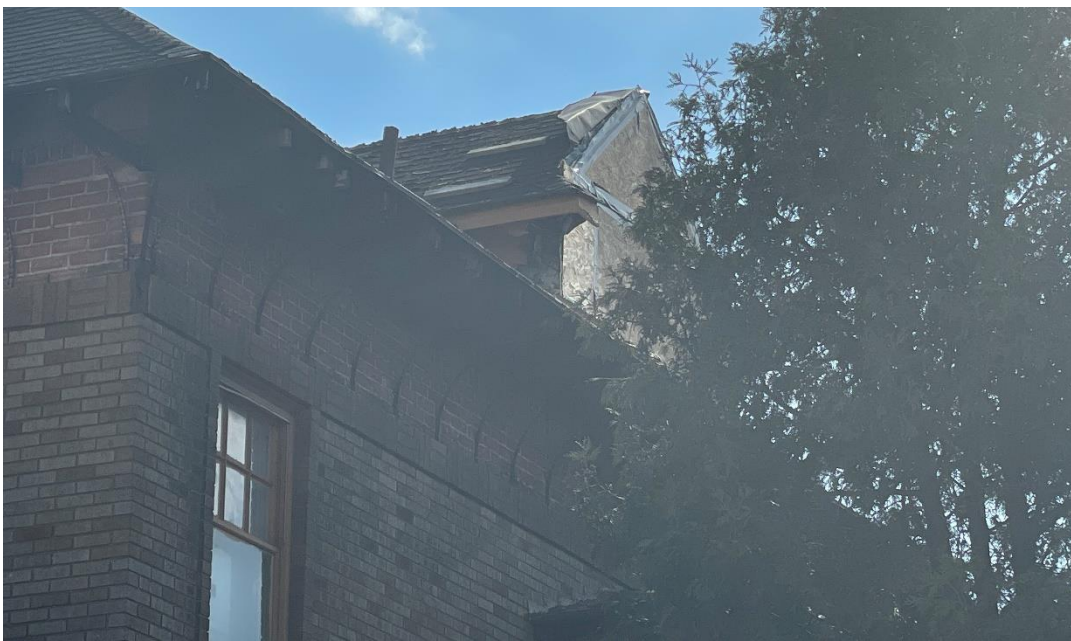
Photo taken by HDC staff in 3/2022 to illustrate unapproved removal of stucco from the side/west elevation dormer
