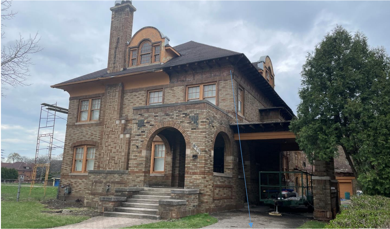
Photo taken by HDC staff in 4/2021 to illustrate unapproved removal of soffit
