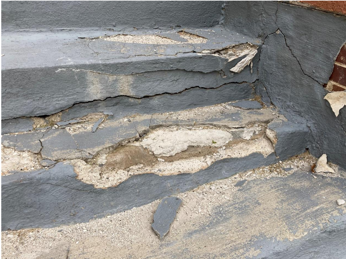
Current conditions at steps. Note thick layer of cement which covers the steps (staff photo taken 10/6/2022)
