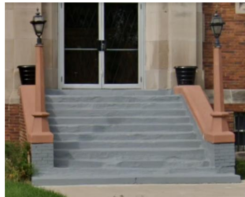
2018 appearance, note cementitious coating has been added to repair deterioration
