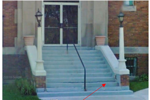
2011 appearance, note cracked step
