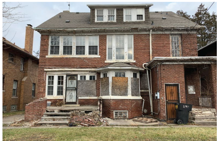
Site Photo 5, by Applicant Jan 2021: (Southeast) rear elevation showing previous windows.
