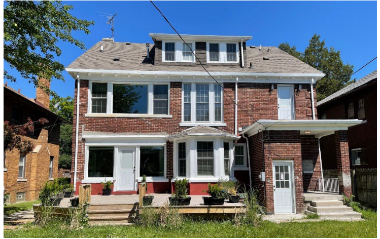
Site Photo 6, by Applicant: (South) rear side elevation showing replaced fiberglass windows on first and second floors and original wood windows on second (middle) and third floors.
