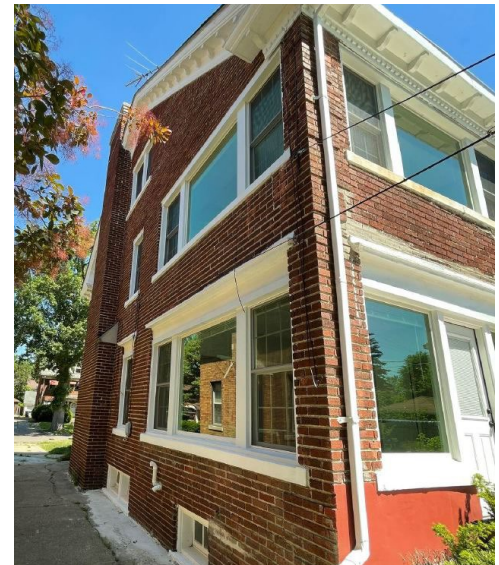
Site Photo 8 by Applicant: (West) side elevation showing fiberglass picture and double hung windows that replaced the original ribbon of wood, double-hung windows on the first and second floors.
