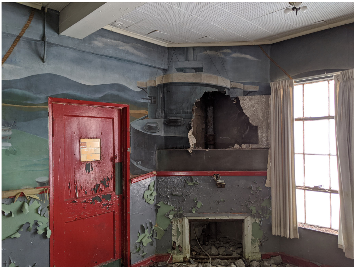
Damage to an area of the Yaeger mural. Staff photo, 2/14/2020.
