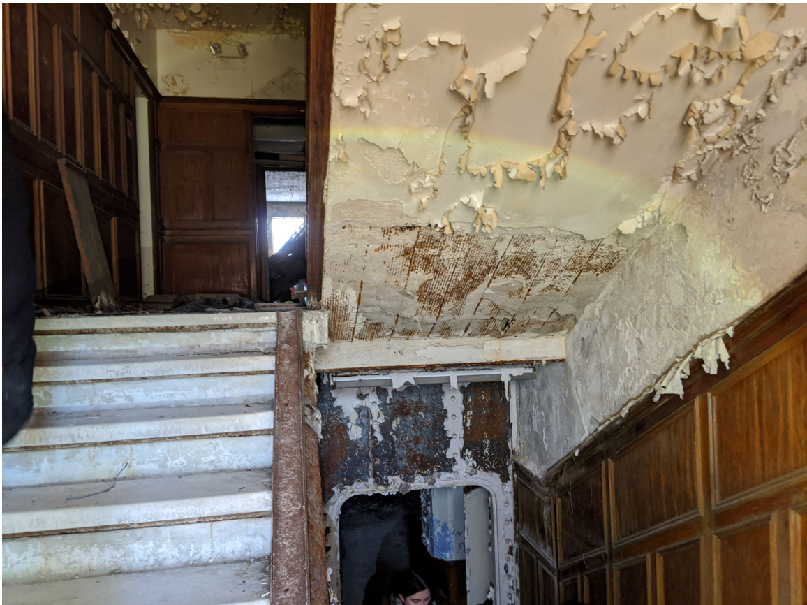
View of stair hall finishes and general condition at south block. Steel bulkhead door visible at bottom. Staff photo, 2/14/2020.
