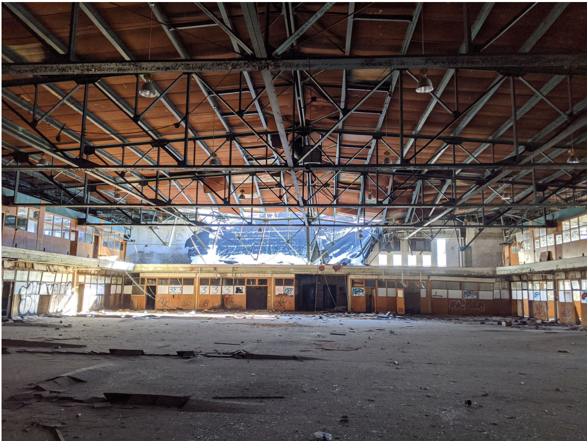
View to south of main drill hall, north block, showing collapsed truss and roof damage at rear. Staff photo, 2/14/2020.
