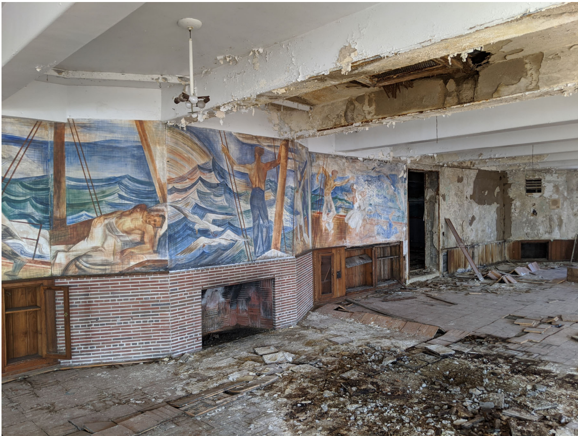
General view of the wardroom and portions of the Fredenthal mural, with water damage towards rear (east). Staff photo, 2/14/2020.
