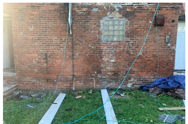
Site photo 5, by Applicant, (Northeast) rear elevation, showing proposed location for stairwell (two boards) and basement door (white outline).
