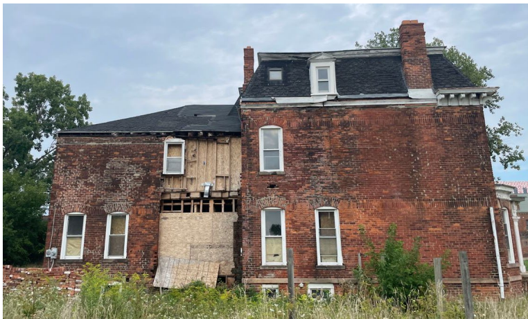
Site photo 2, by staff, August 25, 2022: (Northwest) side elevation showing brick wall, window and door removal locations.
