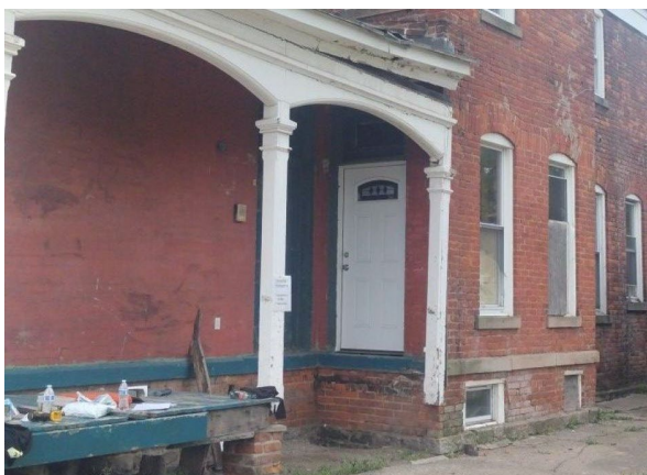
Site photo 4, by applicant: (East) side elevation showing new replaced door and portion of wood porch removed (work done without approval).
