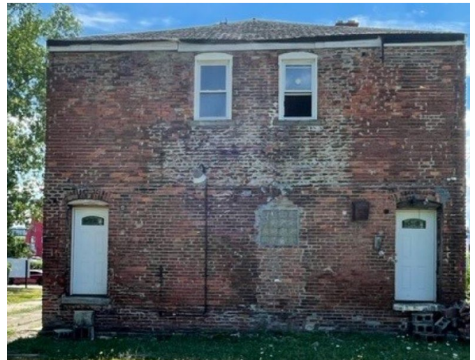
Site photo 3, by Applicant, (Northeast) rear elevation, showing location for proposed balconies, doors and decks.
