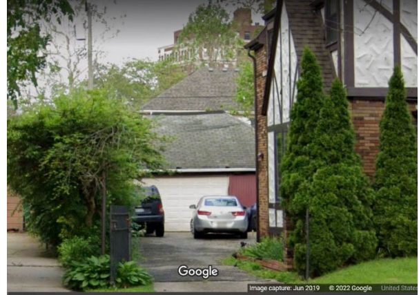
Site Photo 3, by Google Street, June 2019, prior to demolition (by previous owner) of garage showing roof sag.
