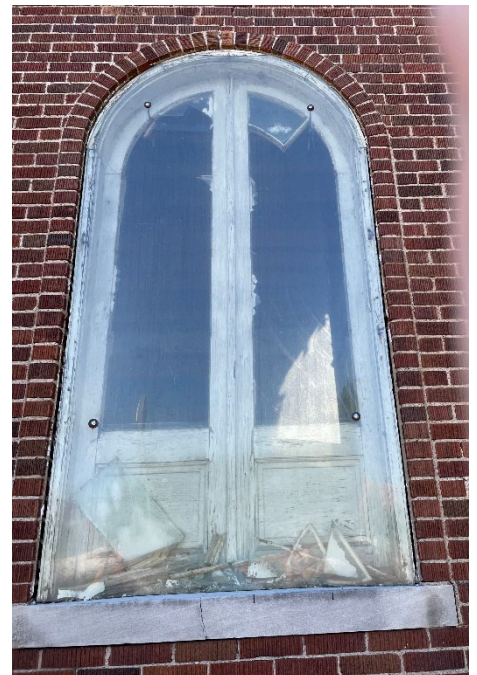
Site photo 4, by Staff July 21, 2022: Side (west) elevation showing condition of existing wood door/windows: while the radial pattern of the divided light is mostly lost, the wood structure of the door and its paneling is intact.
