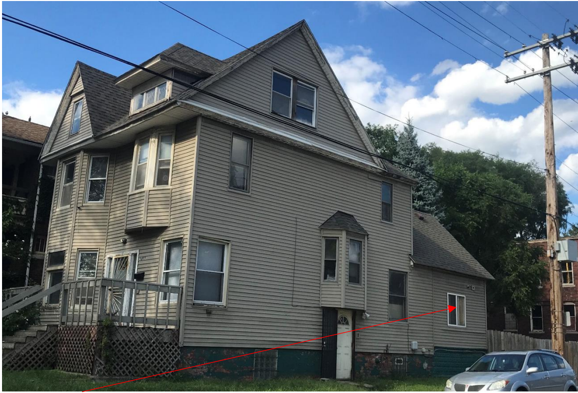
Vinyl windows at rear enclosed porch, HDC staff photos dating from 2020, prior to the unapproved work.
