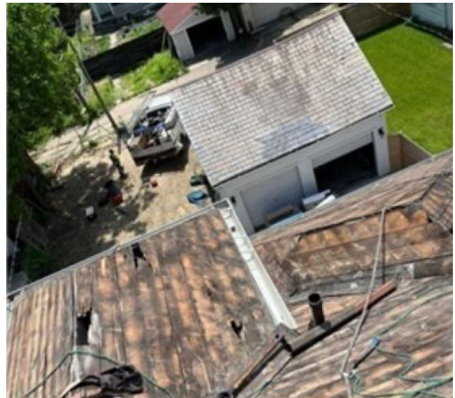
Site photo 6, by applicant: (Southeast) rear elevation of roof showing conditions of the roof after slate removed. The garage’s slate roof is visible in the background.
