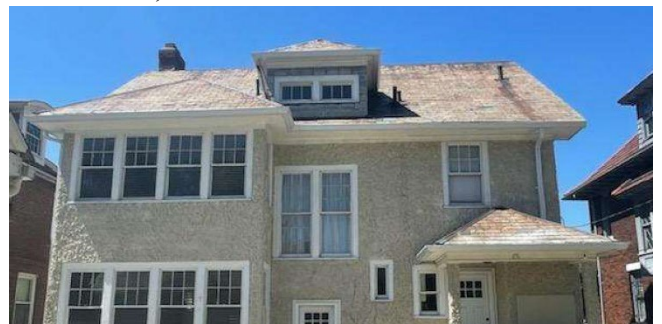
Site photo 5, by applicant: (Southeast) rear elevation of roof showing conditions of slate roof.
