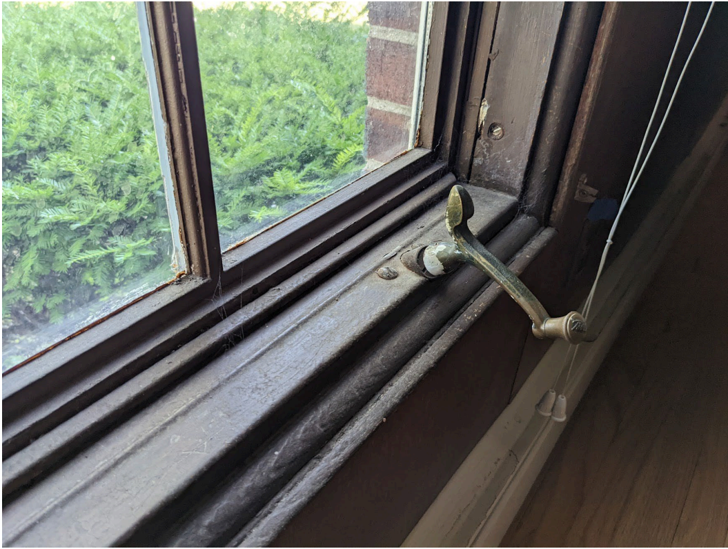
View of window with operator crank intact. Staff photo, July 12, 2022
