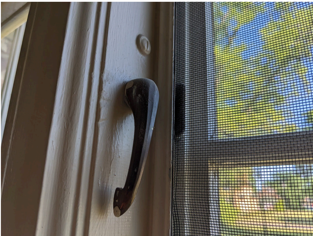
Typical view of ornamental closer at mullion, one of two per sash. Staff photo, July 12, 2022
