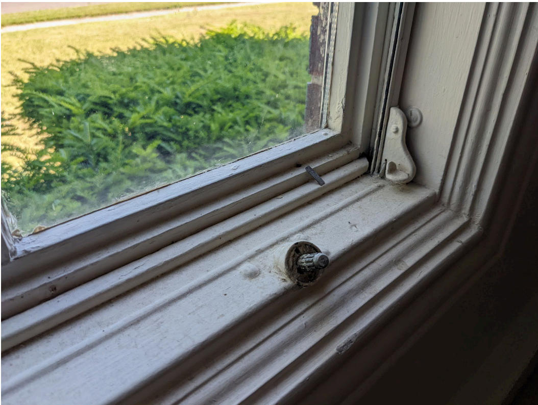
Interior detail view of typical sill conditions. Note missing operator, worn spline, and insulated glazing. Staff photo, July 12, 2022
