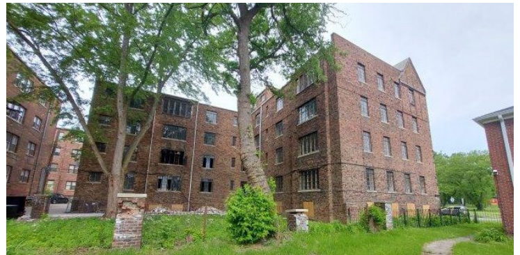
Site Photo 2 by Applicant: (Southeast) rear elevation, showing fire damage on east-facing, rear wing of the building.
