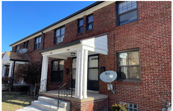
Site Photo 2, by Staff February 24, 2022: (Southwest) front elevation on Manderson, showing vinyl window installation.
