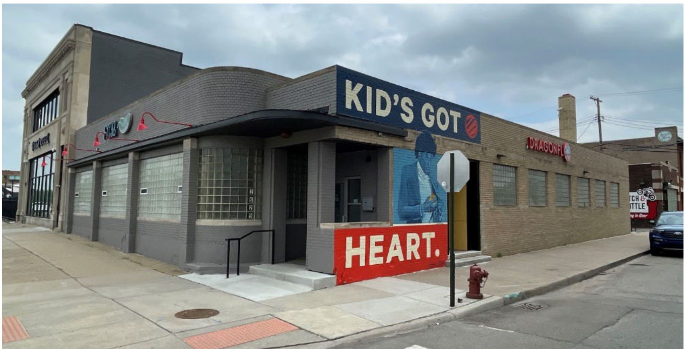
Site Photo 1, by Staff May 20, 2022: (Northwest) Front elevation at the corner of East Grand Blvd and Beaubien St., showing unapproved painted brick in grey (on the left) and mural, and the proposed buff brick (on the right) to be painted in grey to match.
