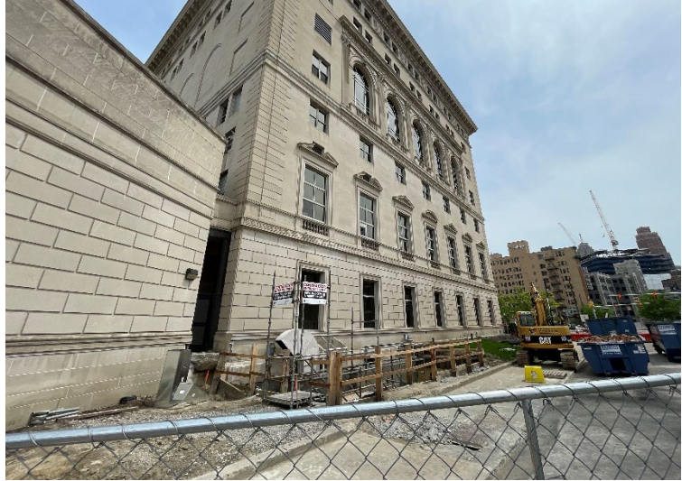
Site photo 3, by Staff, May 20, 2022: (West) side elevation looking south, showing work along stairs to basement and temporary removal of staircase.
