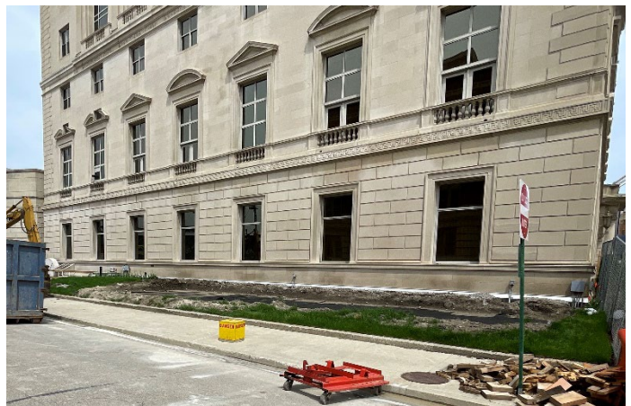
Site Photo 2, by Staff May 20, 2022: (West) side elevation on John R, showing proposed site work has broken ground.
