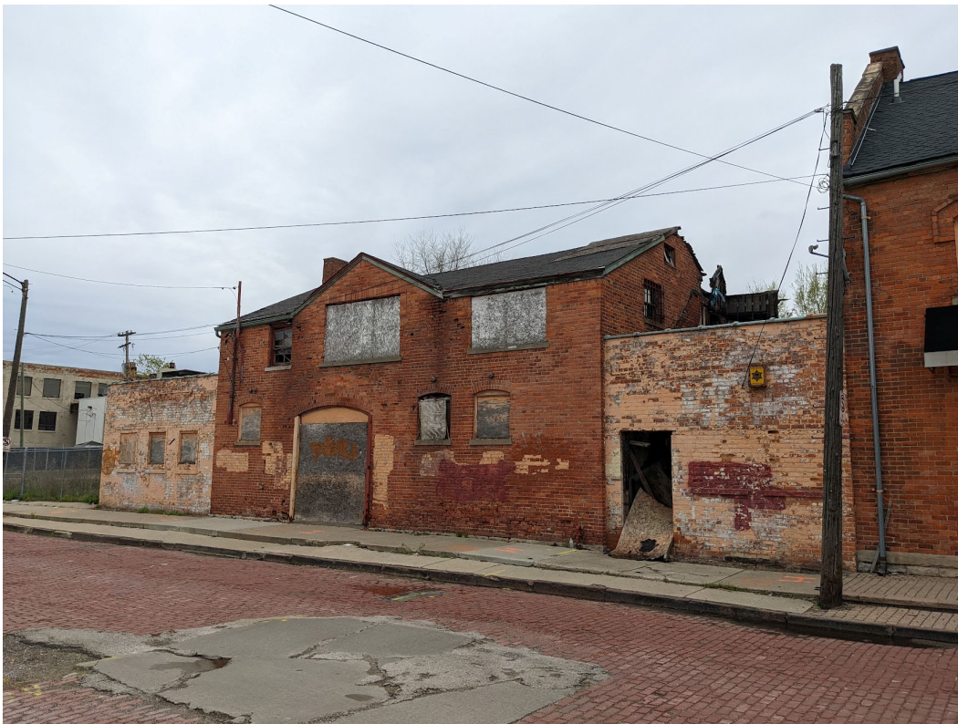
View of existing conditions at 1977 Woodbridge. Oldest portion at center (2 stories, unpainted brick). Flanking 1-story buildings are the painted brick additions at either side. Historic district building at far right of image (see photo on page 2). Staff photo, May 6, 2022.
