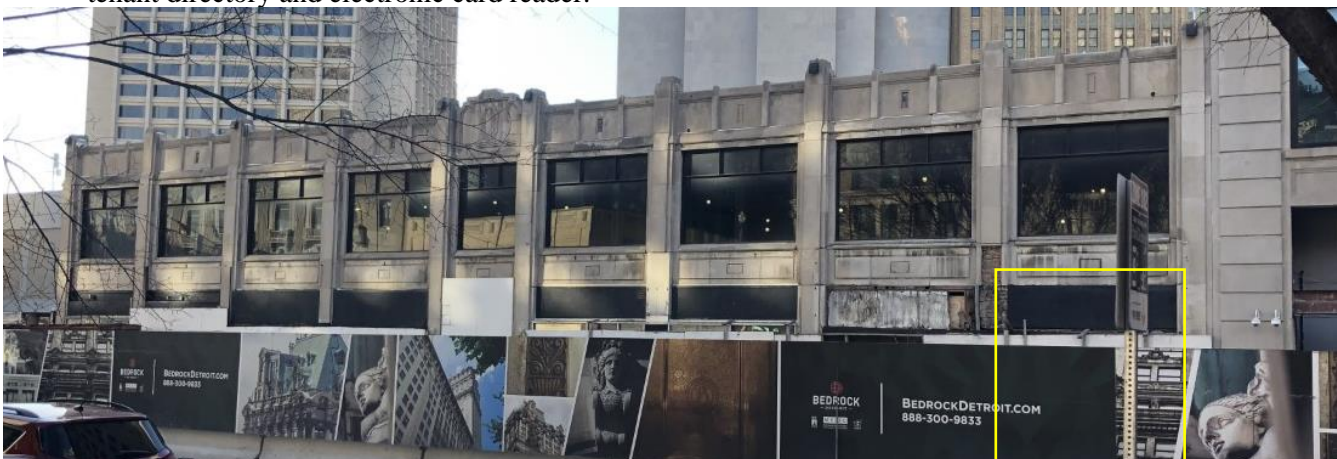
North elevation, storefront opening that will become a recessed entry is highlighted. Staff photo, January 29, 2021.
