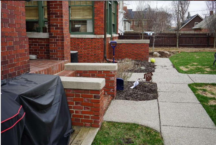
Photo 8 View of two back stairs looking south showing that the sunroom stairs is two feet longer and extends to the sidewalk Also shows proximity of the sunroom .
