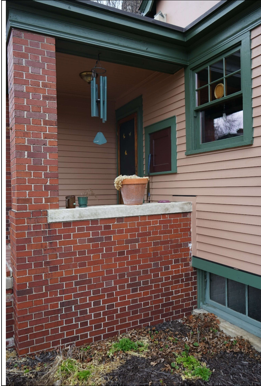
Photo 6 Back porch from south showing where wall will be built on top of Limestone cap. Proposed window will be at same elevation as the existing window in pantry. Remaining wall will be clad in matching wood siding.
