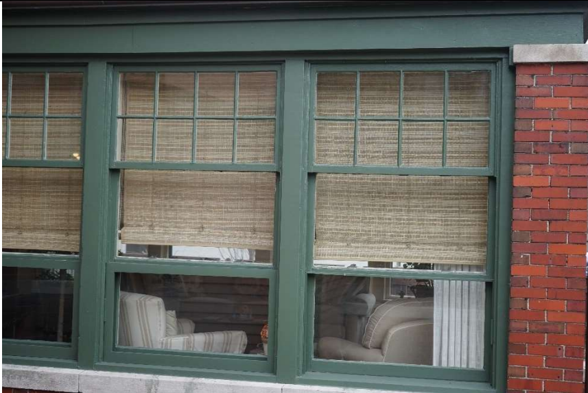
Photo 7 Sunroom window, new window will match the upper sash muntin pattern and be similar in size
