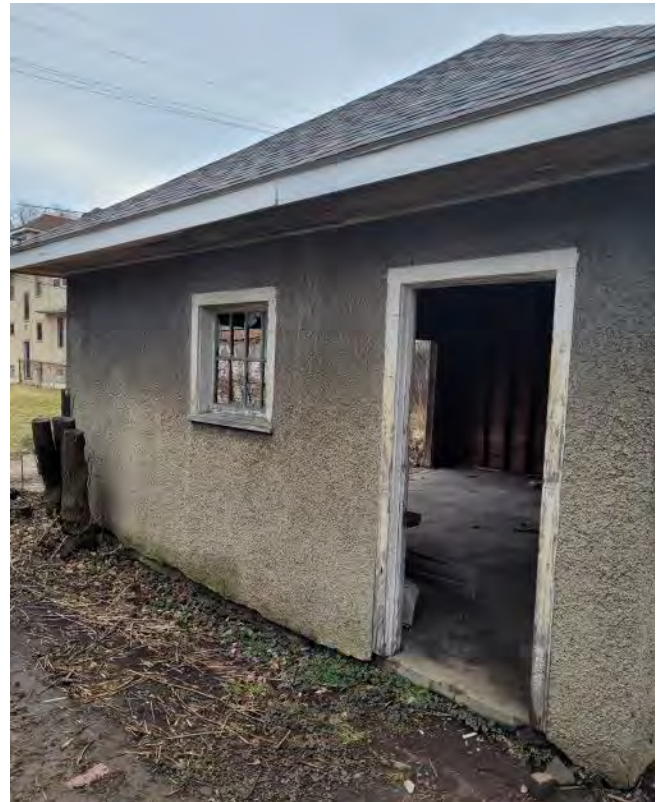
Site photo 3, by Applicant showing garage at the rear of the property with new asphalt roof (work completed without approval).
