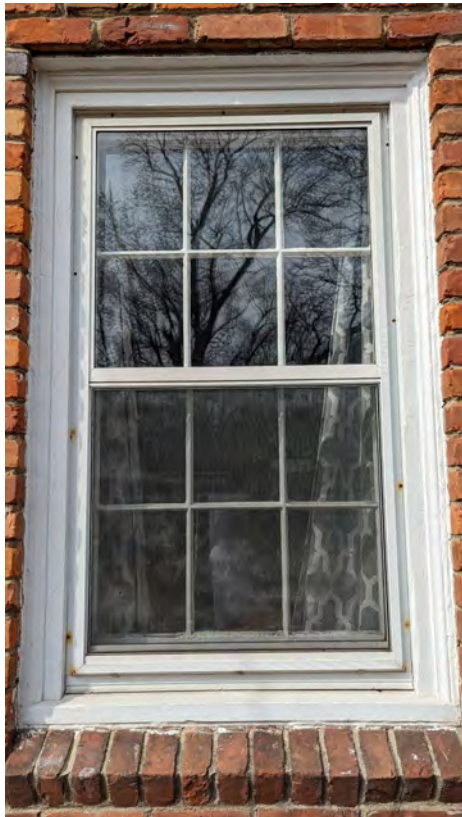
8. exterior view rusting frame and fasteners
