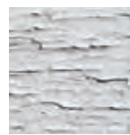
REAL WOOD Peeling, Rotting, Pests, Mold
