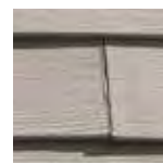
FIBER CEMENT Cracking, Fading, Off-Gassing
